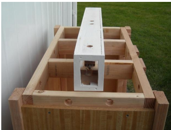
End where Ground Fault Duplex goes
